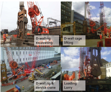
Machinery that will be used on our streets to construct the new deeper cutting
