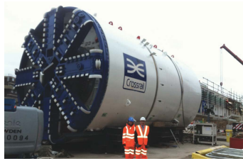
Two tunnel boring machines will arrive at the new portal south of Parkway
